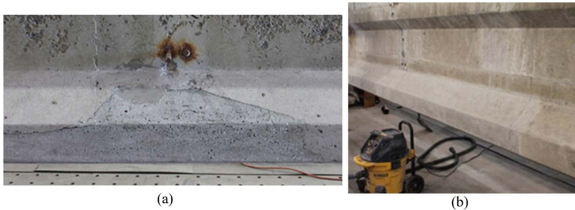
Figure 26. a) Repair Location after Formwork Removal b) Repair Location after FRCM Surface Preparation
