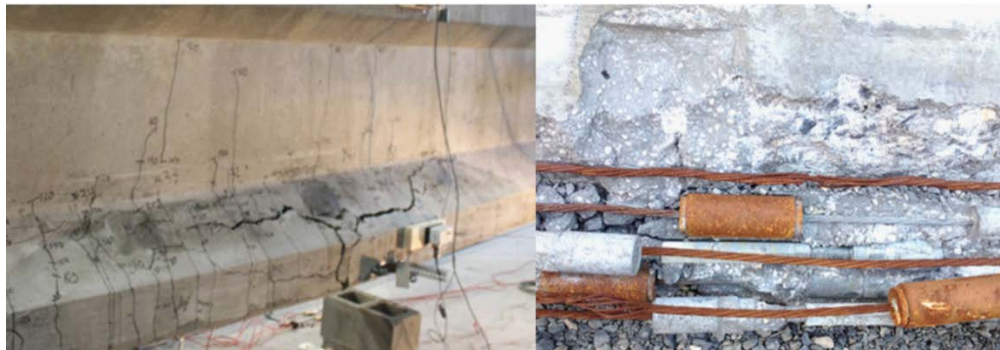
Figure 53. Flexural Cracks in Patch Concrete at Failure (left) and Failed Splices and Strands (right)
