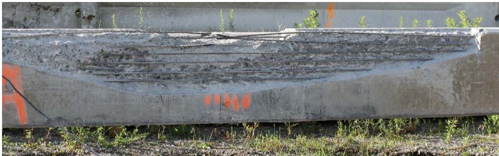
Figure 20. Damage Location for Test 4 Before Repair
