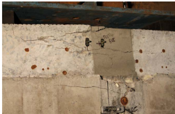
Figure 60. Compression Failure in the Composite Deck
