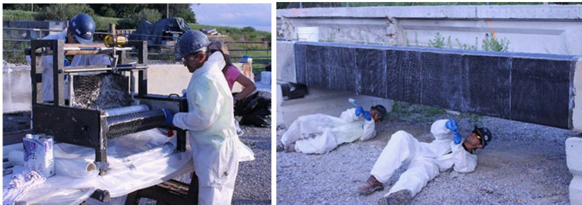
Figure 23. Fiber-Reinforced Polymer Saturation Process and Rolling of FRP Fabric to Ensure Bond to Concrete
